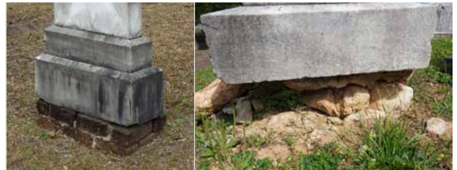
(Above Left) Brick foundation. Flemington Presbyterian Church, Liberty County. (Above Right) Rubble and fieldstone foundation. Oakland Cemetery, Fulton County.
